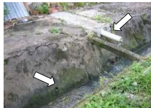
Plate 1: Black water outlet (left channel) and grey water (right channel) outlets to storm water drain in central Kuching
